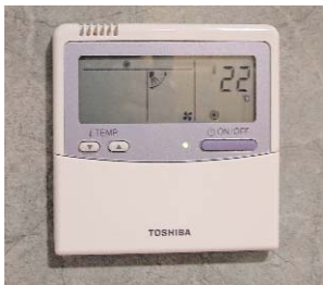
The room controllers are neat and easy to understand
